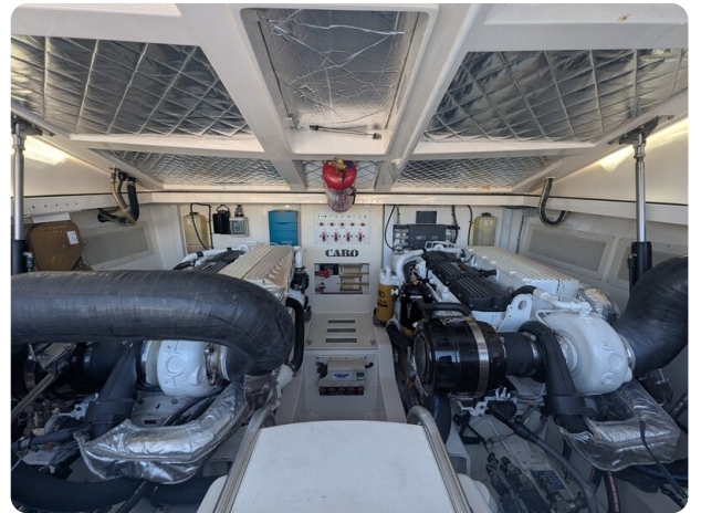
Cabo 38 Express engine room
