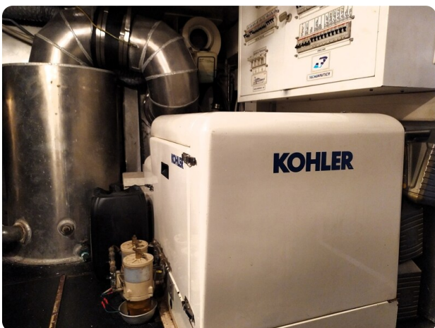
SANLORENZO SL 62 Generator
