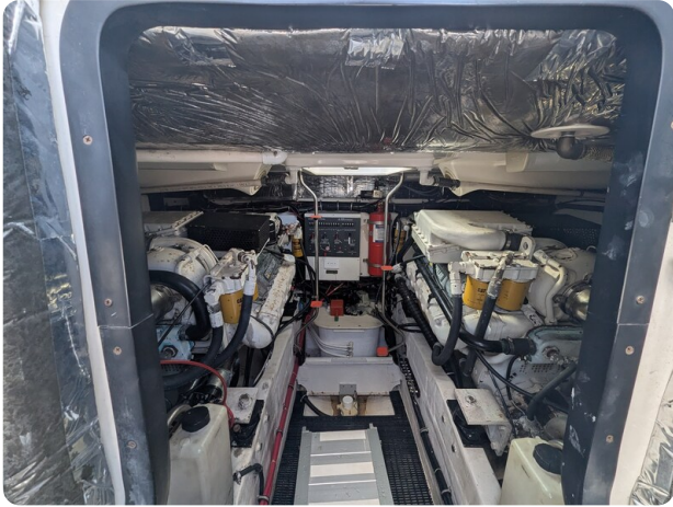
Tiara 4100 Open engine room
